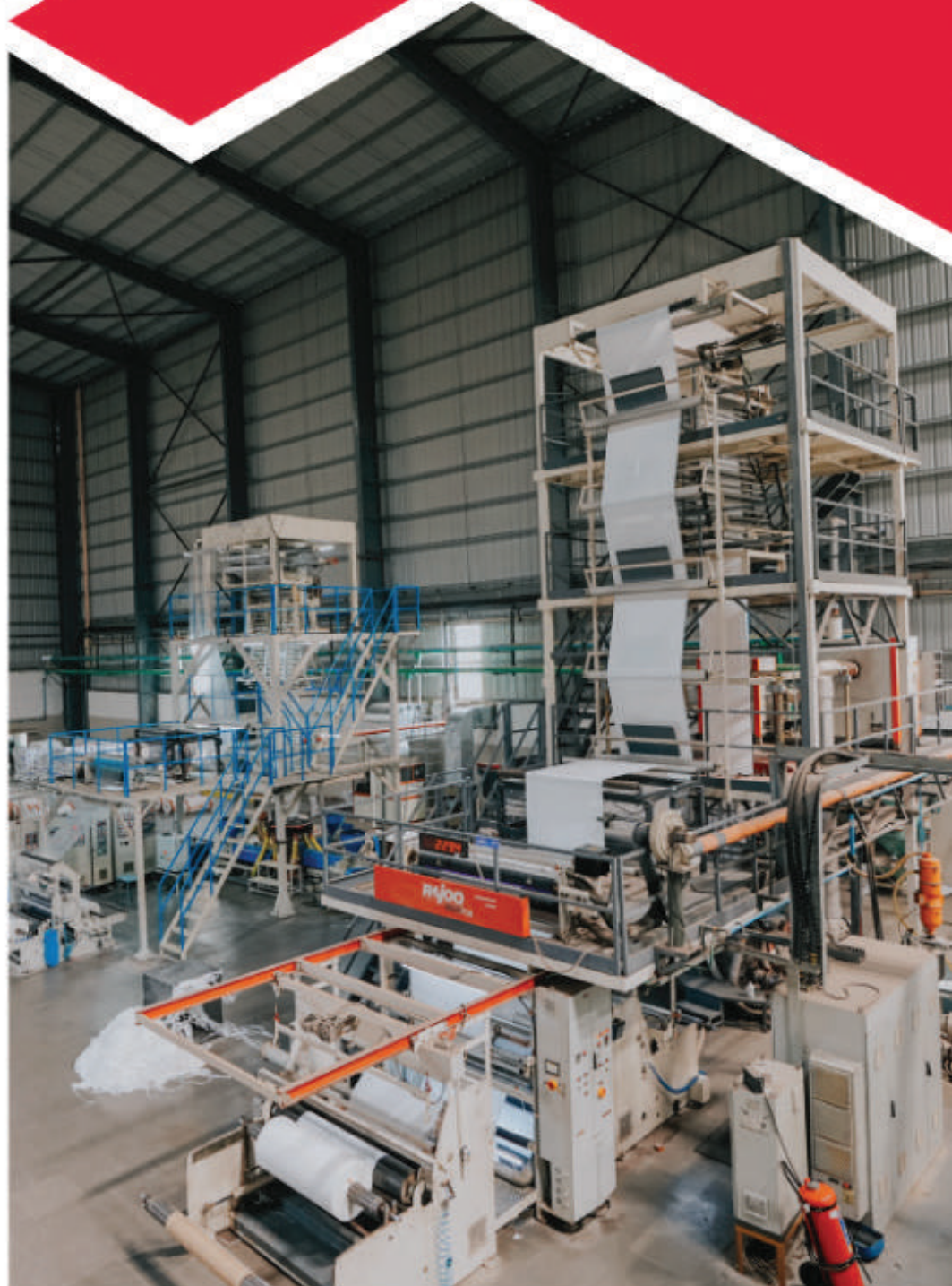
3 LAYER BLOWN FILM PLANT WITH IBC AND PLAST CONTROL
